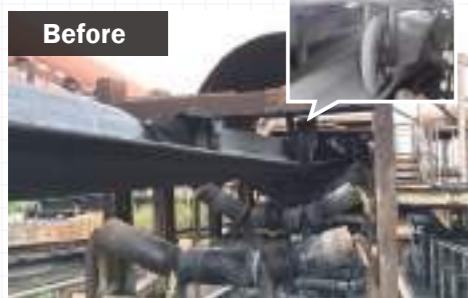
The belt was forcibly pressed down by the wheels, causing belt damage and contributing to mistracking.
