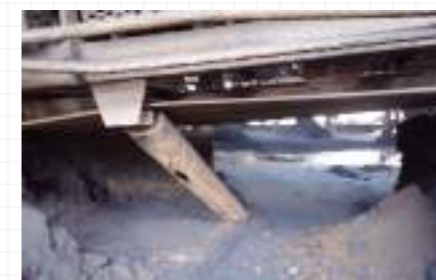
Belt mistracking causes bulk material spillage, leading to higher cleaning costs and increased material loss.
