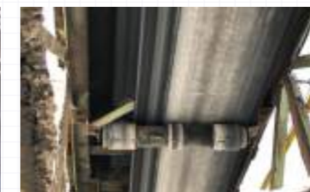
Frequent emergency stops due to belt misalignment detectors lead to a significant decline in productivity.
